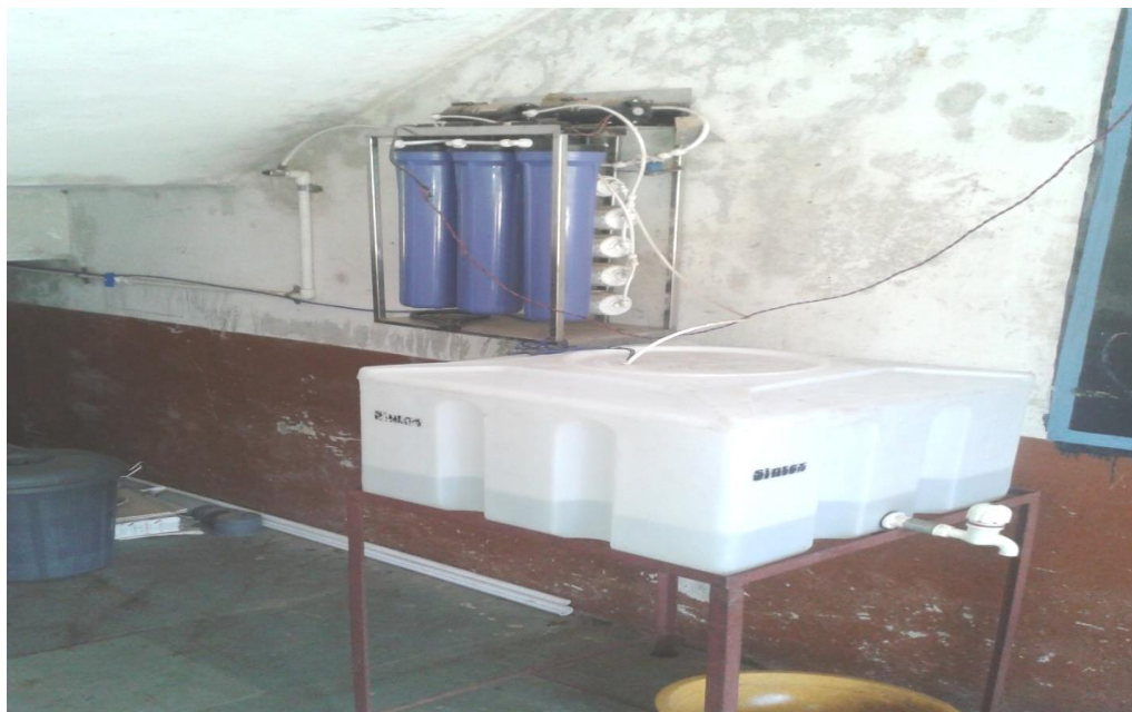
Drinking water: R.O plant purifier water
